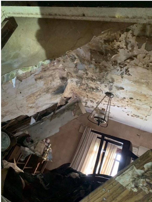
Second-floor water damage.
