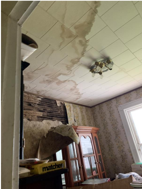
Main floor water damage.
