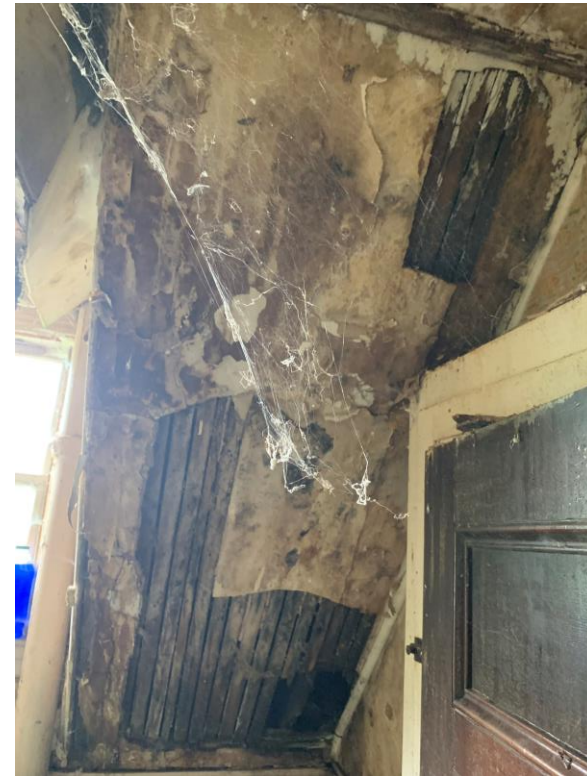
Second-floor water damage.
