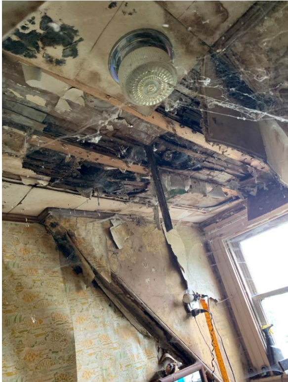
Second-floor bathroom water damage.
