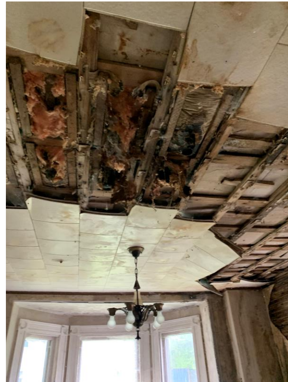
Main floor water damage.
