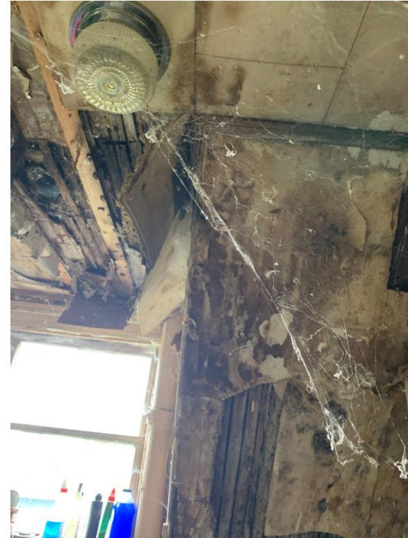
Second-floor bathroom water damage.
