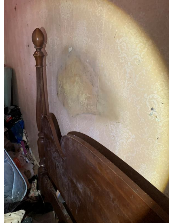
Second-floor bedroom. Light appeared to scorched wallpaper.
