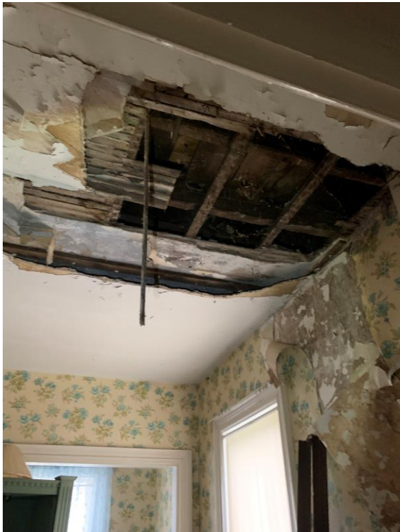
Second-floor water damage.
