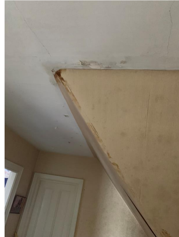
Minor water damage on second-floor.
