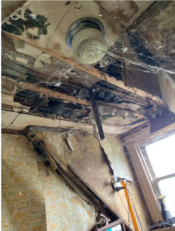
Second-floor bathroom water damage.
