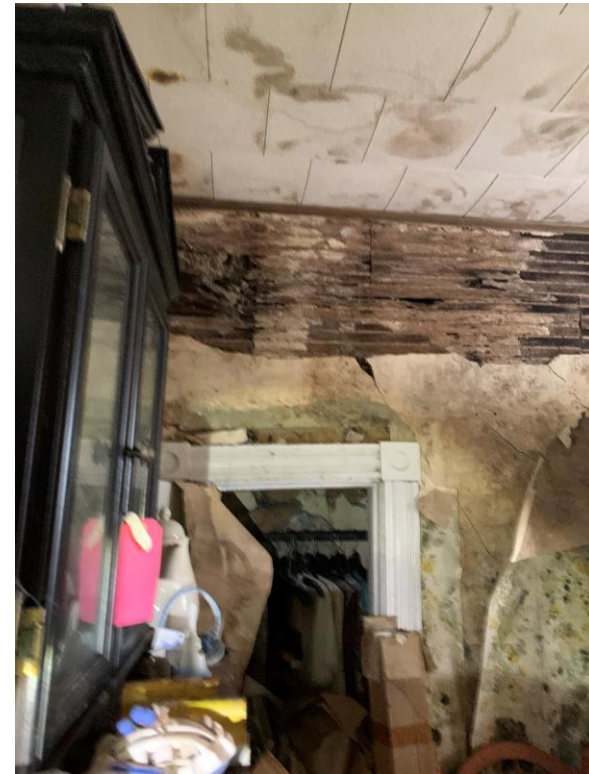
Main floor water damage.
