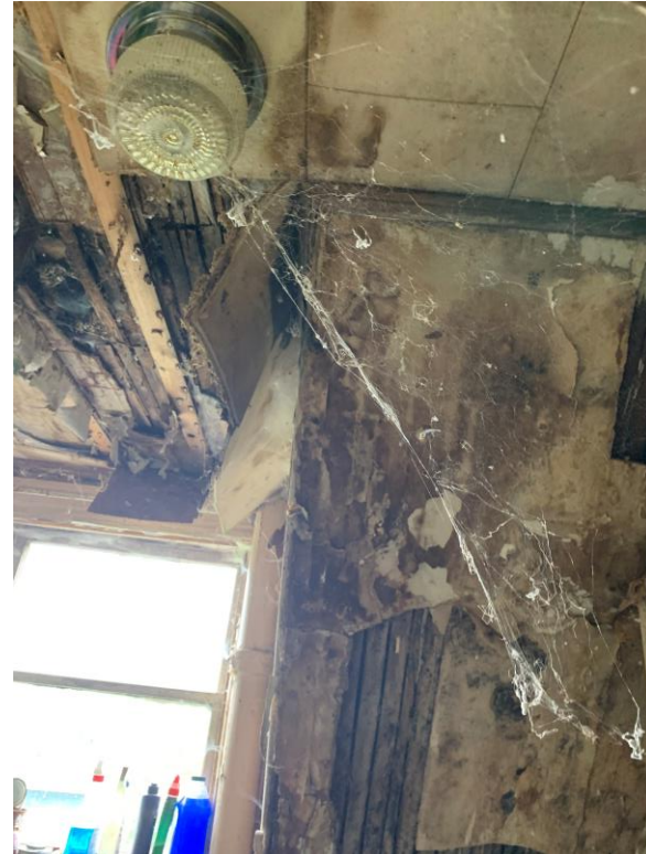
Second-floor bathroom water damage.
