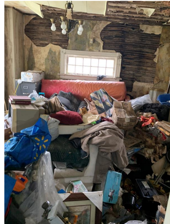
Main floor water damage, hoarding.
