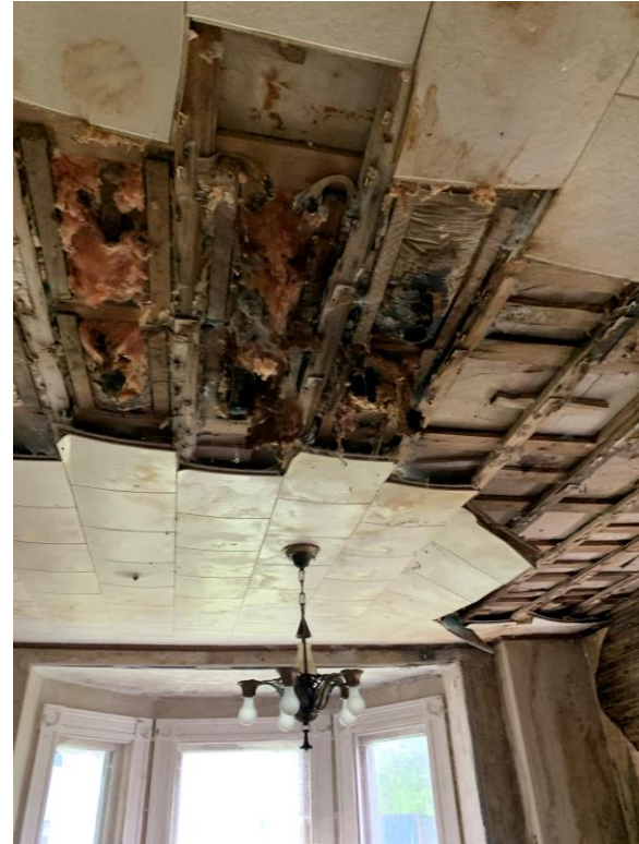
Main floor water damage.
