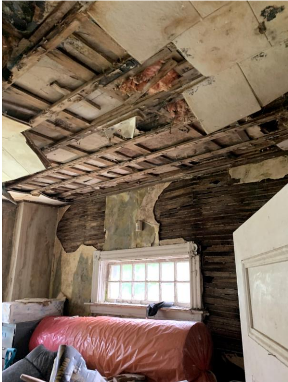
Main floor water damage.
