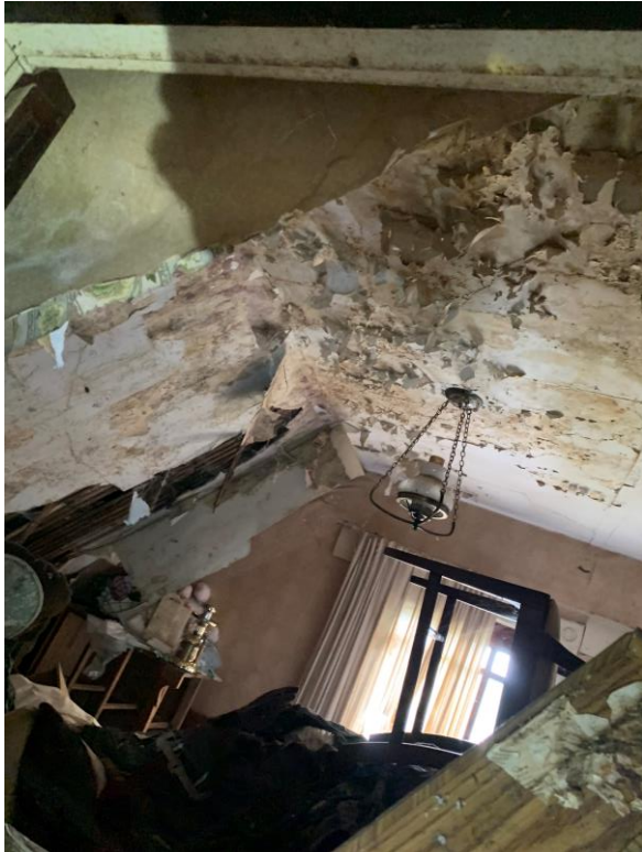
Second-floor water damage.
