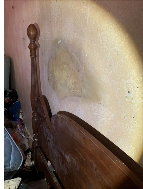
Second-floor bedroom. Light appeared to scorched wallpaper.
