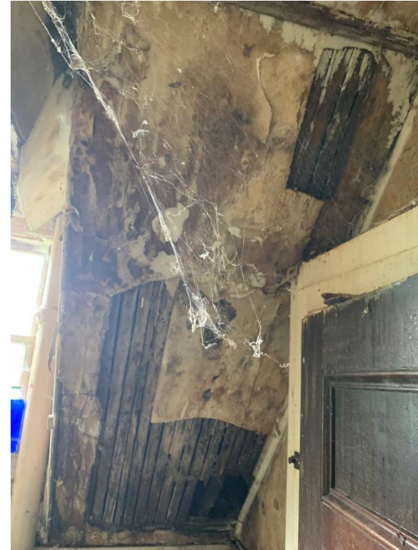
Second-floor water damage.
