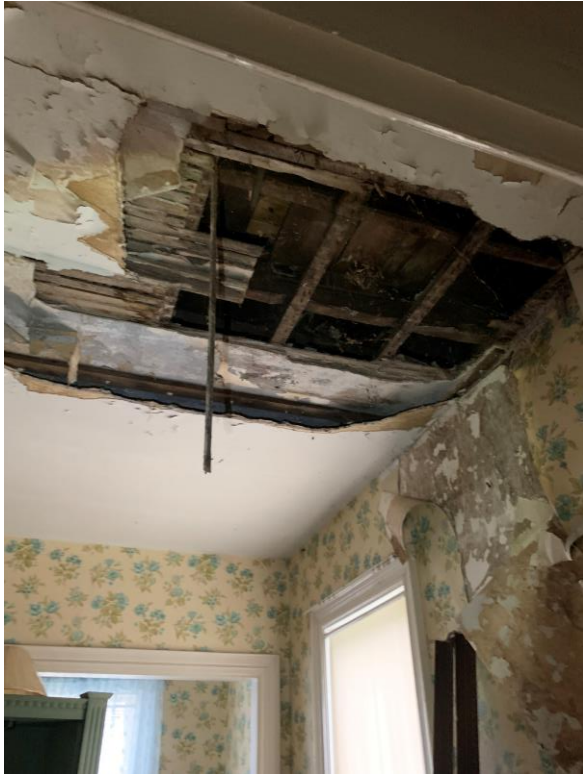
Second-floor water damage.
