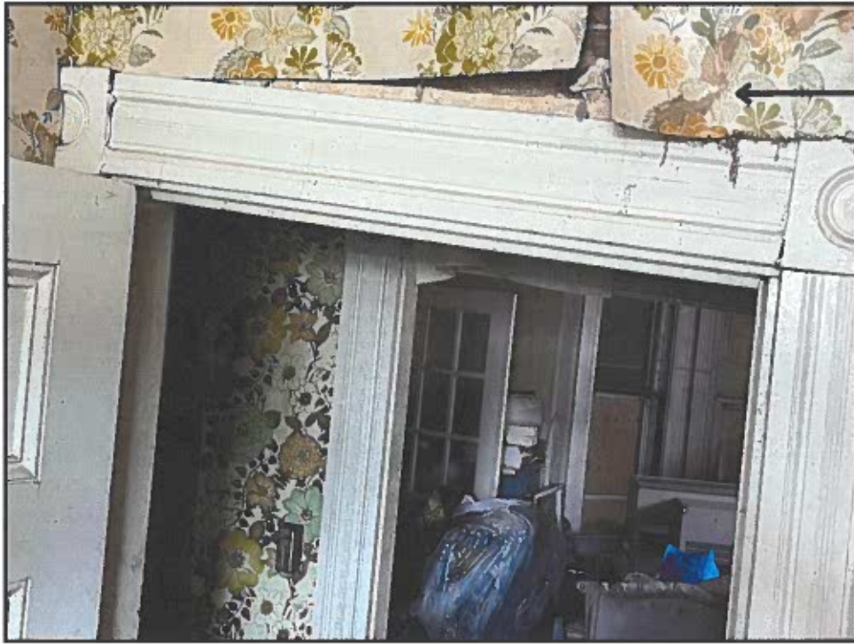
Slanted door frame due to active settlement. Approximately 3 1/2" of settlement in a 3'-0" run
